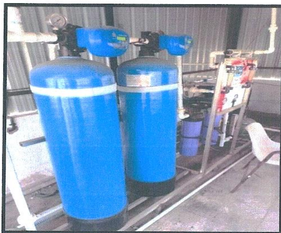
Sewage Treatment Plant
