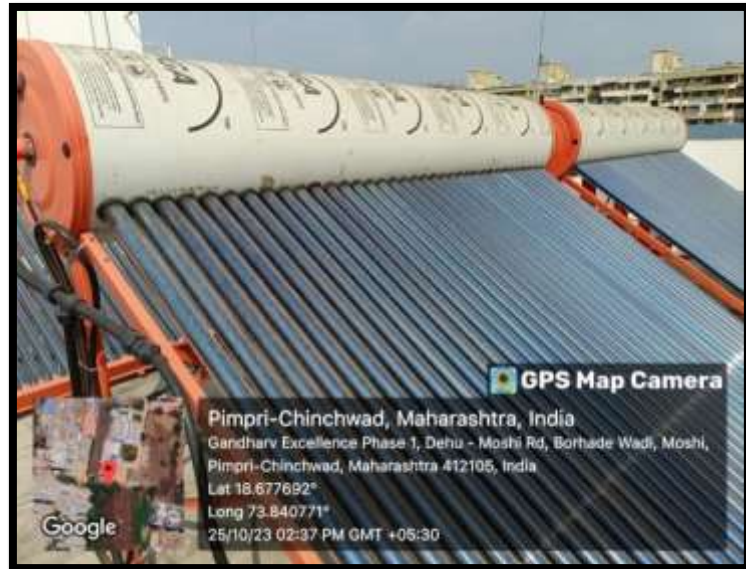
Solar Water Heaters
