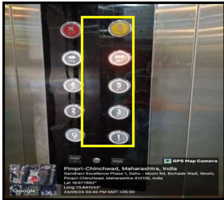
Disable Friendly Lift Facility
