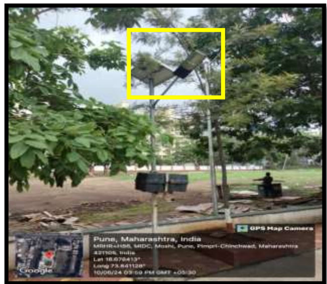
Solar street lamp
